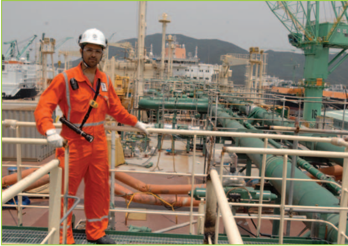
Abdullah on the main deck of one of the vessels under construction
